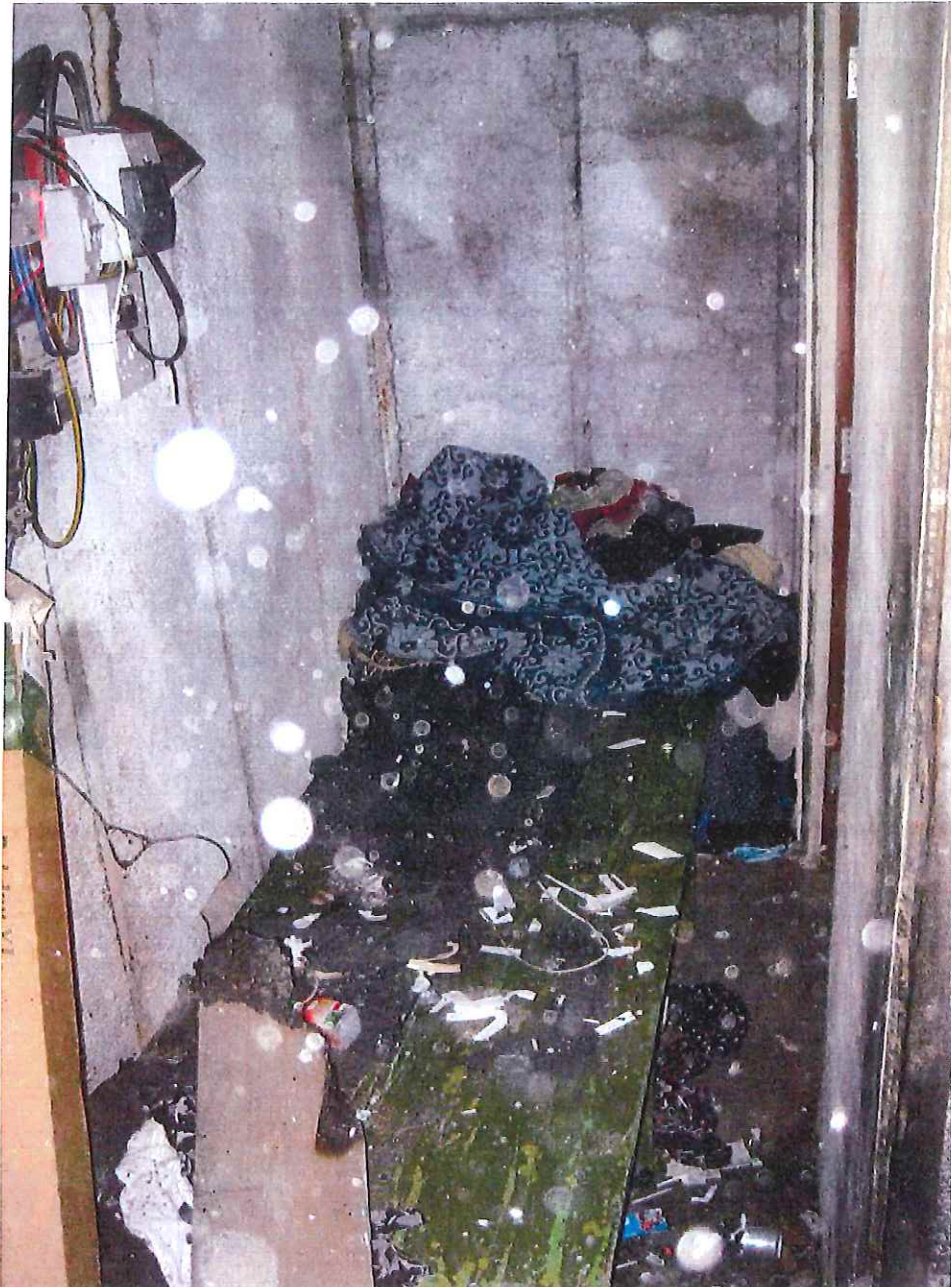
Fig 8. Evidence of someone sleeping rough in pavilion.
