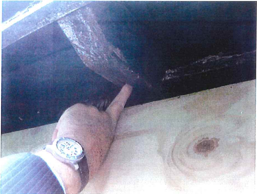
Fig 7. View of severely decayed rafters.
