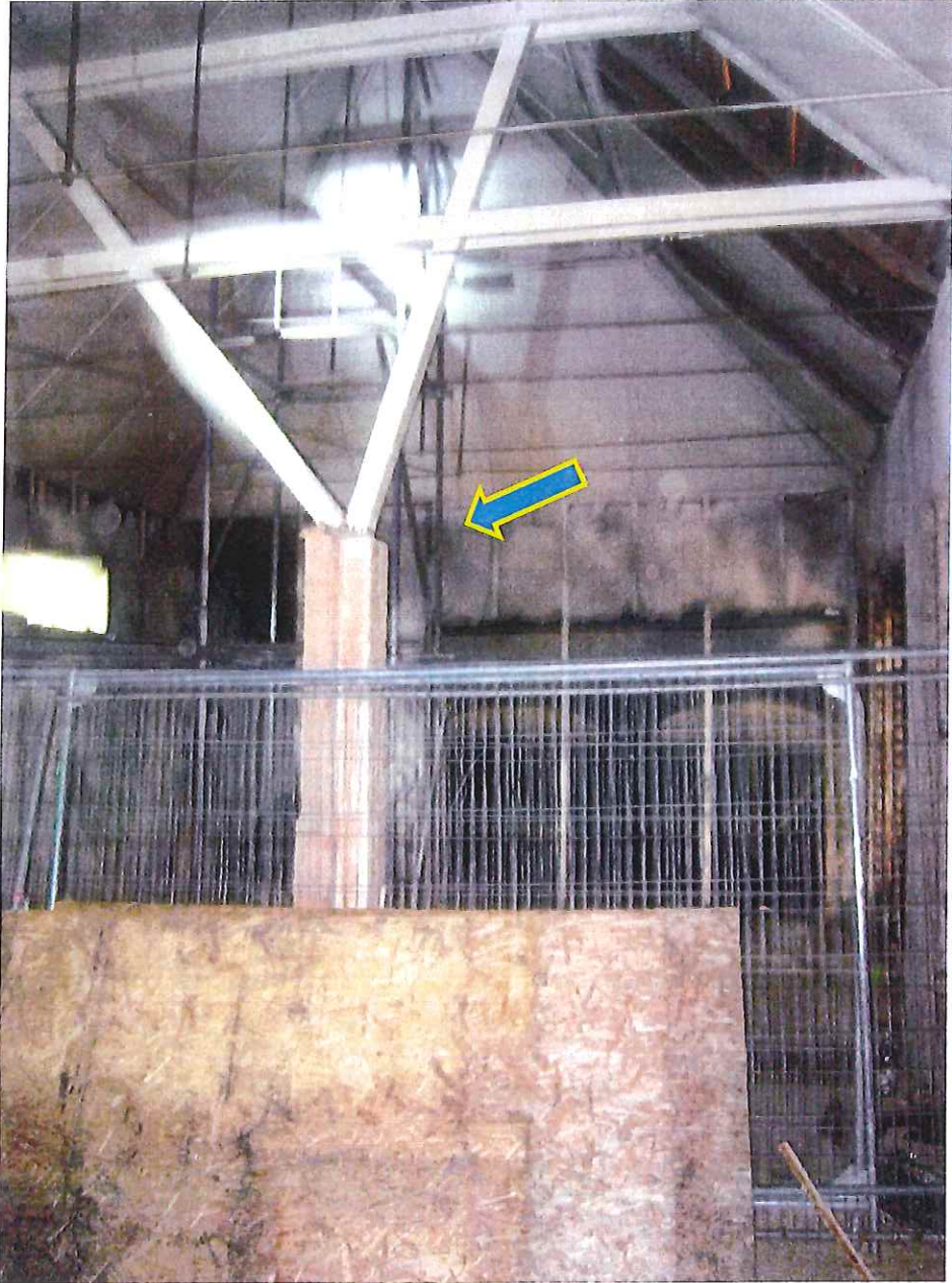
Fig 4. View of central brick pillar with main roof truss members sat on top.
