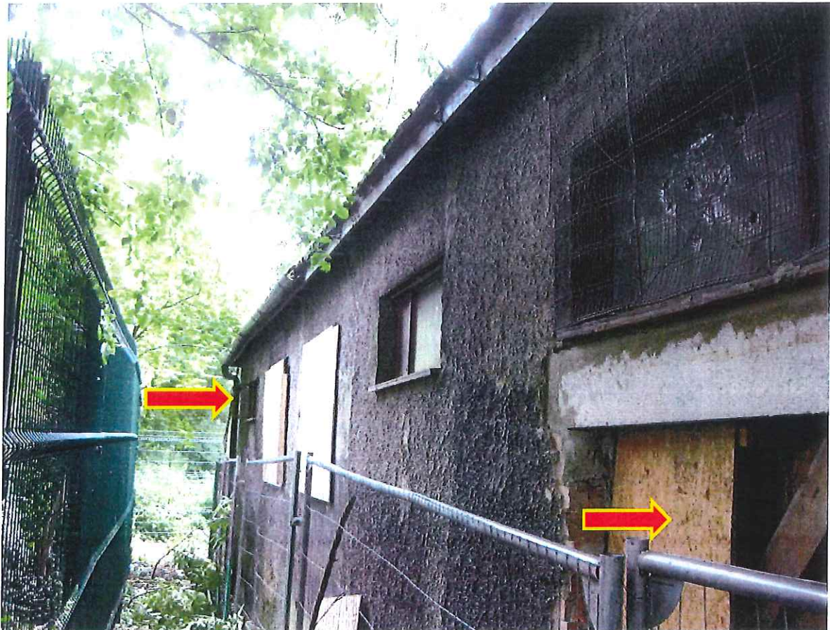
Fig 7. Rear of building insecure. Hole knocked in rear wall by existing tenant and window removed.
