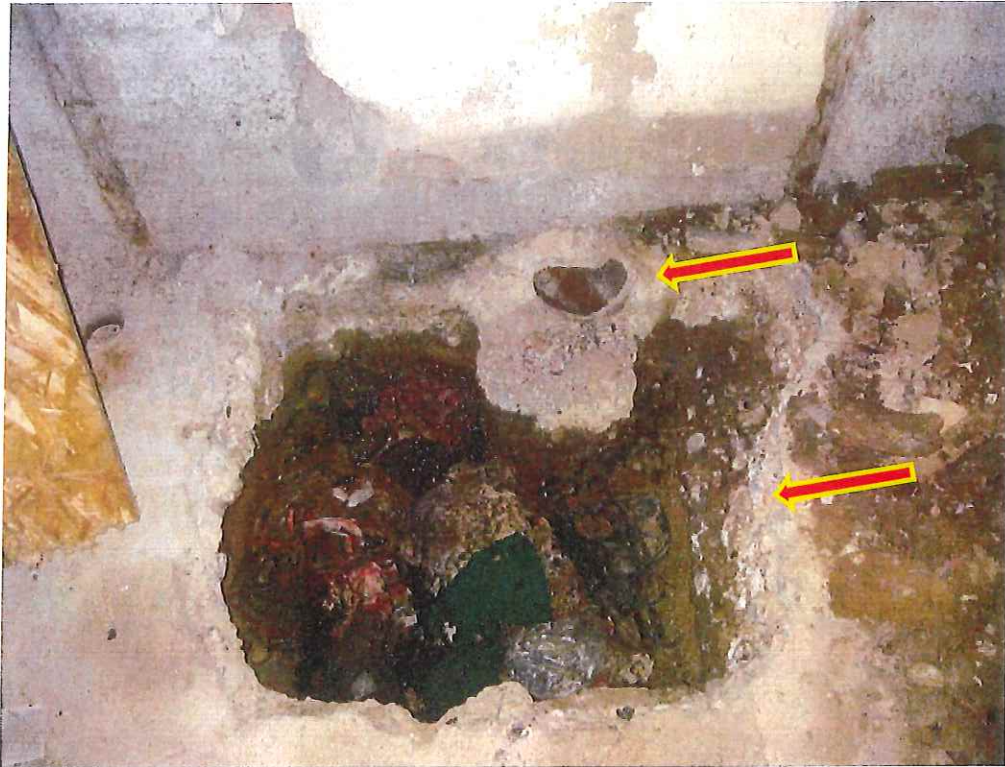
Fig 12. There are several holes in the floor. The holes appear to be trial pits to check out ground conditions below the concrete floor slab. There are also open drainage connections within the building.
