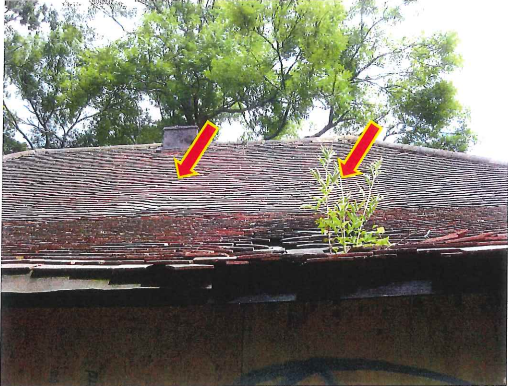
Fig 5. View of roof from front of the building, note the areas sagging caused by decay and lack of appropriate support.
