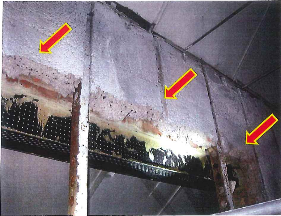
Fig 9. Unsupported concrete panels between corroded metal studs could collapse. This is typical of several locations.
