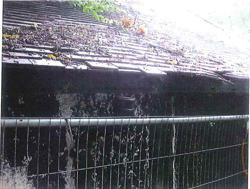
Fig 6. View of roof from side of the building, note the areas sagging caused by decay and lack of appropriate support.
